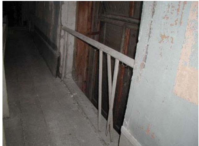
Figure 71. At one time, railings with 3/4" square balusters were inset into each of the tall window openings at the gallery level. They functioned as guardrails and should be reinstated according to the remaining evidence.
