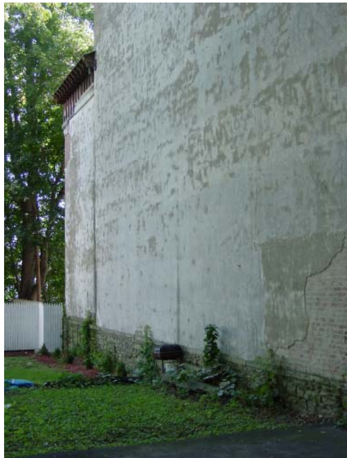
Figure 18. North elevation. Note delaminated rendering exposing brick structure and overgrown vegetation.
