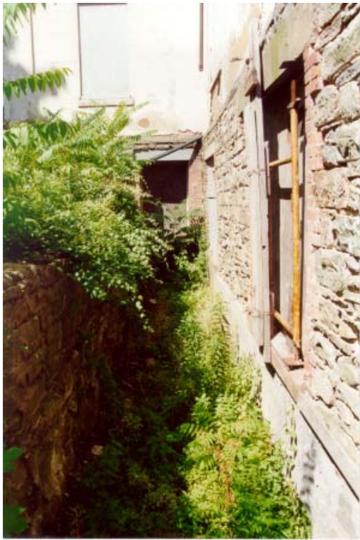
Figure 16. West Areaway, note the jacks supporting lintel in window opening and cementitious parge coat along base of wall.
