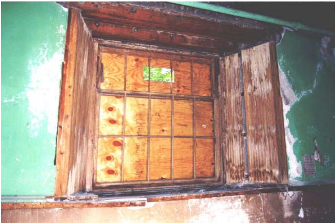
Figure 44. The basement window at northwest corner of Sessions Room is the only example in situ of the historic sash and frame likely original to the building. Note the modern wood headers installed to stabilize the opening. The beaded board is likely not original to the Davis design of the building. The deep recesses open onto the Areaways to the east and west.
