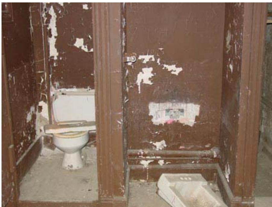
Figure 72. Ladies toilet stall located under the Portico. None of the plumbing is functional at this time.
