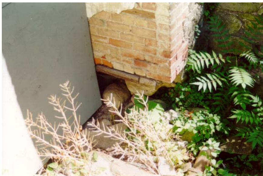
Figure 15. Base of foundation wall deteriorated with large portions of missing stone in west areaway.
