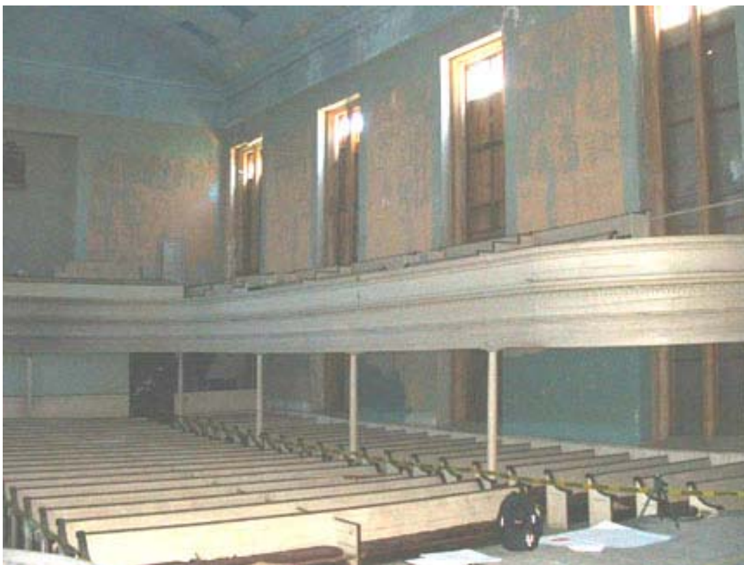
Figures 55 and 56. View of west wall of Nave and gallery (above) Note the peeling paint layers that expose the 1906 stencil pattern (below).
