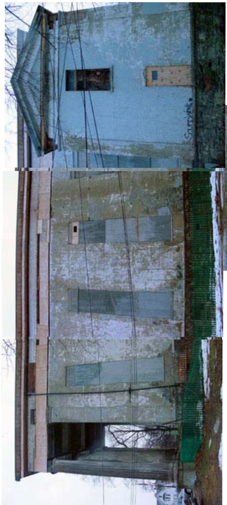
Figure 23. Collage of east elevation. Similar problems persist on the other long elevation of the Church, however, the wall has not subsided. Note the plywood covering the window openings and the spalling of the lime rendering,
