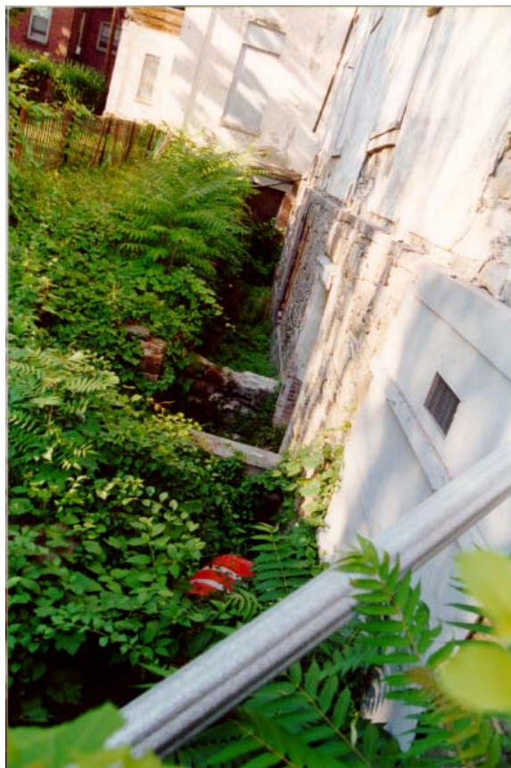
Figure 14. West areaway looking north. Note excessive vegetation overgrowth and boarded window and door openings.
