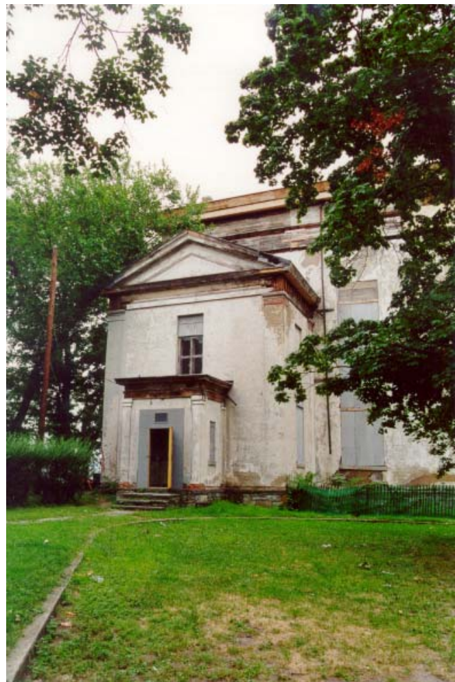
Figure 34. West transept and entry. Note the missing portions of the entablature and the missing lime-based rendering that reveal the brick structure beneath. The brick masonry is indicative of the 1867-8 additions. The door has been removed and placed in storage.
