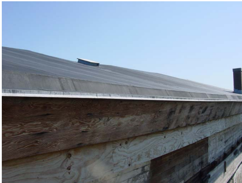
Figure 33. View of the EPDM roof installed in the 1980s during the tenancy of the Hudson Valley Freedom Theatre. The temporary plywood gutters are largely ineffective, as leaders have become detached and water runs into the Areaways below. Note the saddleback in the roof at the hatch location. Further investigation into structural movement will be necessary to determine the appropriate treatment for the problem.
