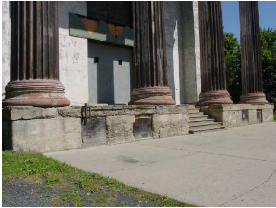
Figure 19. Deteriorating concrete at south elevation portico. Column shafts have no paint coating to protect exposed wood from ultraviolet deterioration.
