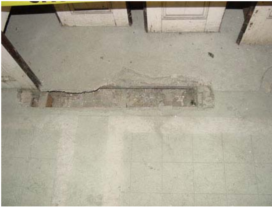
Figure 53. The framing for the infill is visible due to the damage to cementitious flooring in the Nave. The aisle floors were scribed to mimic a tile pattern.
