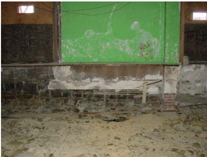
Figure 47. The east wall in the Sessions Room is typical of the deterioration of the plaster walls and footings in the basement.
