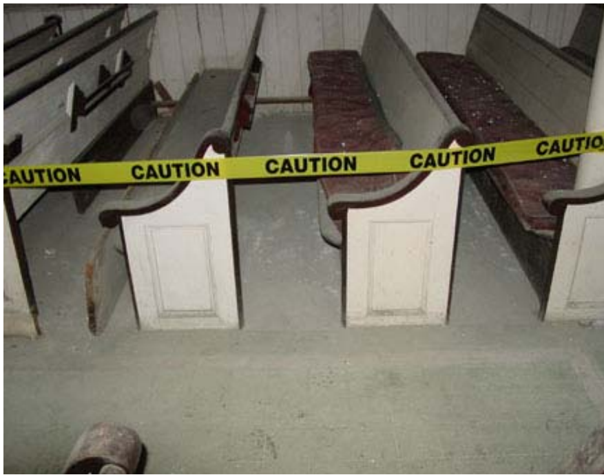
Figure 54. The pews along east wall of Nave. Two iterations of the design exist in the building and can be identified by the molding profiles in the panels. Their bases have been submerged in the cementitious material to varying levels due to the settlement of the floors. Dutchman repair of the wood at the bases of the pews will be necessary as well as general stabilization and repair on those more damaged. Paint analysis, stripping, priming and repainting/restaining are all required.
