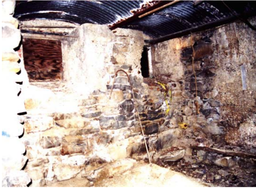
Figure 50. View of the interior of south wall beneath the Portico illustrating the deteriorated condition of the steel beams supporting the corrugated metal jack arches installed in 1910. The piers beneath the columns are approximately 4'x4'; the walls between the piers are roughly 18" thick.
