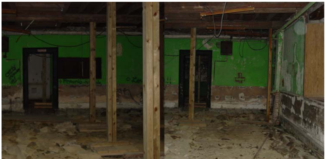
Figure 39. Collage of South wall of Sessions room. In the foreground can be seen the shoring and temporary footings installed by the National Parks Service in 2002 to stabilize the main floor. Note the absence of the floor and the ceiling framing.
