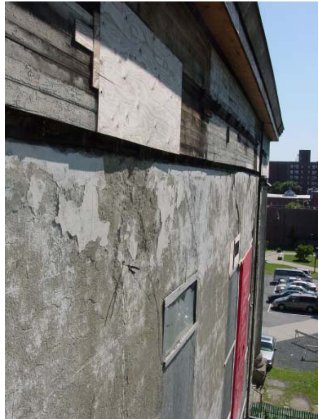
Figure 21. View of west wall looking south. Entablature and rendered façade deterioration. The entablature molding has been removed and stored.
