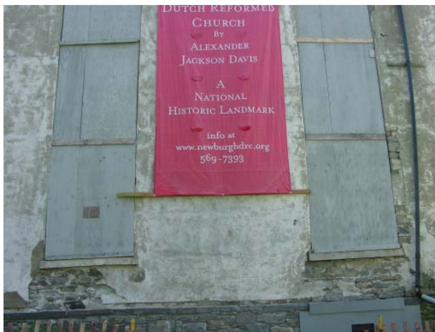
Figure 22. Areas of spalled and missing rendering expose the rubble stone wall on the west elevation allowing for close inspection of the masonry system specified by A.J. Davis..
