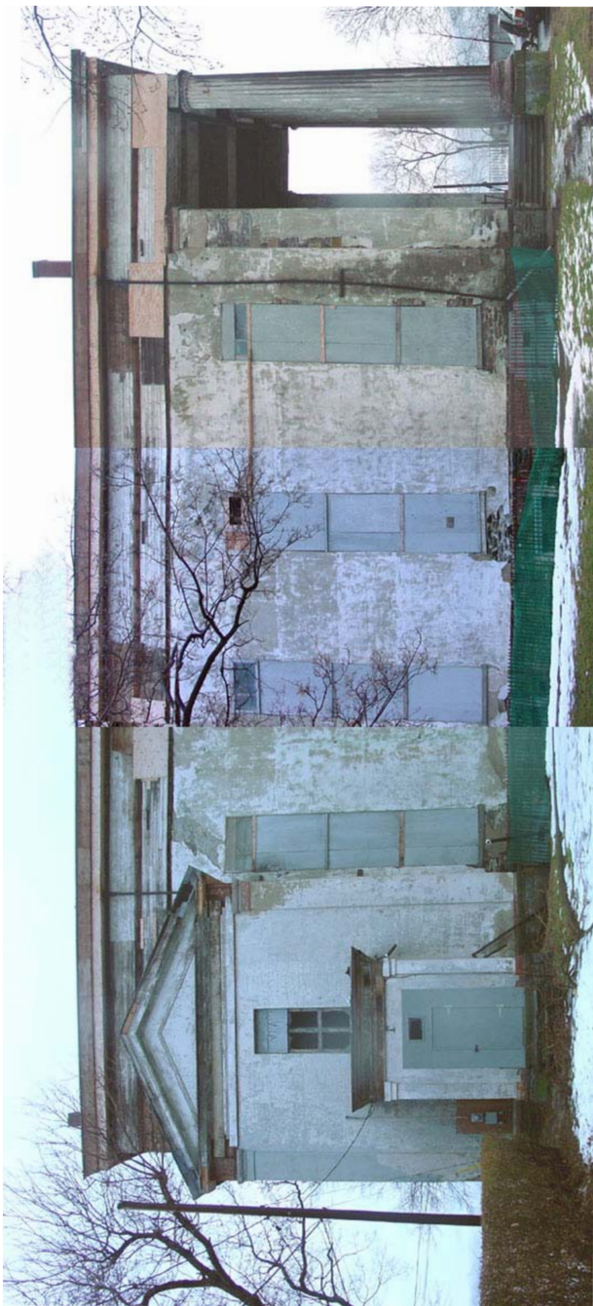
Figure 20. A collage of west elevation illustrates the deteriorated condition of the lime rendering, the subsidence of the center of the wall and the missing entablature elements.
