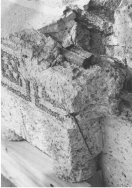
Fig. 9. Cutaway view of taenia, regula, and guttae shows the "before" condition of the decorative surface and corrosion of the embedded steel reinforcing. Photograph by the author.
