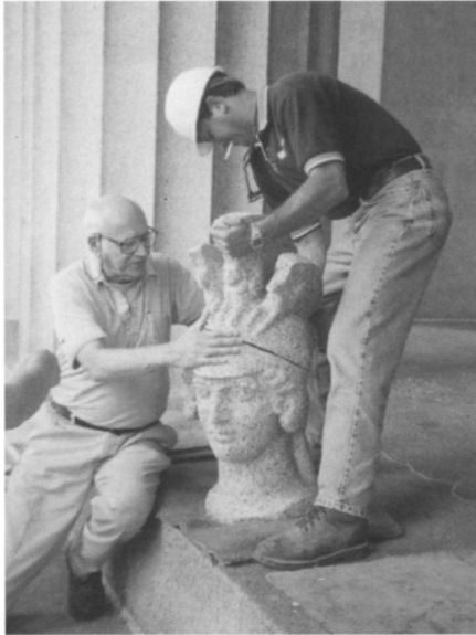
Fig. 7. Dr. Kreier and Ken McAbee from Western Waterproofing test the mating of two pieces of the Athena sculpture before inserting anchoring steel and lifting her into position. Photograph by the author.
