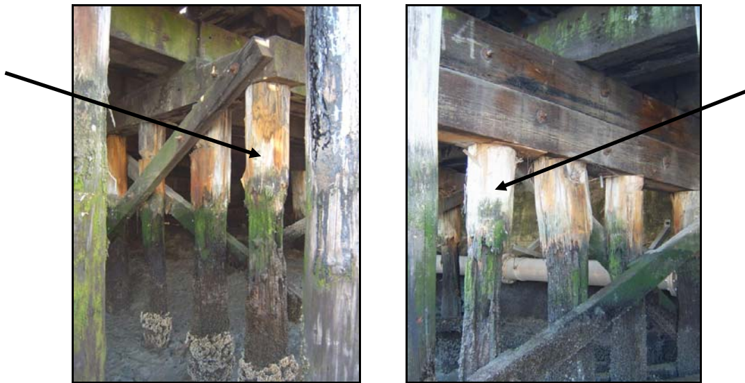
Figures 22 & 23. Photographs representing pile conditions. The rightmost pile in Figure 22 (arrow) is rated “poor,” the pile to its left rated “fair.” The leftmost pile in Figure 23 (arrow) is rated “beyond poor;” the remaining piles visible in Figure 23 are rated “fair.” ( PAST Consultants, LLC Photos )
