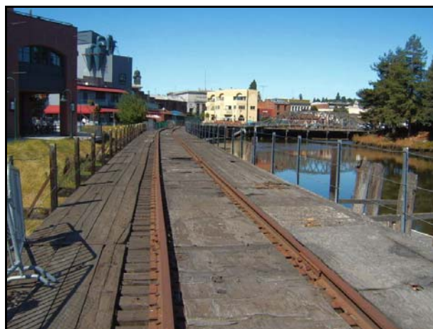
Figure 16. Deck view taken from east abutment. Note the railings, replaced deck boards, and plywood. ( PAST Consultants, LLC Photo )
