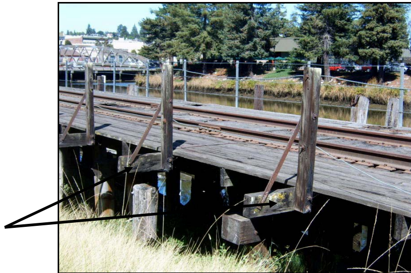
Figure 27. South rail connected to outriggers (arrows). The north rail is mounted to floor joists cut flush with the north face of the structure. ( PAST Consultants, LLC Photo )
