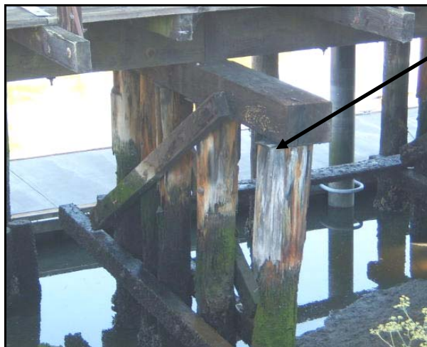
Figure 24. Exposed pile top at interface with bent cap, indicated by arrow. (PAST Consultants, LLC Photo)
