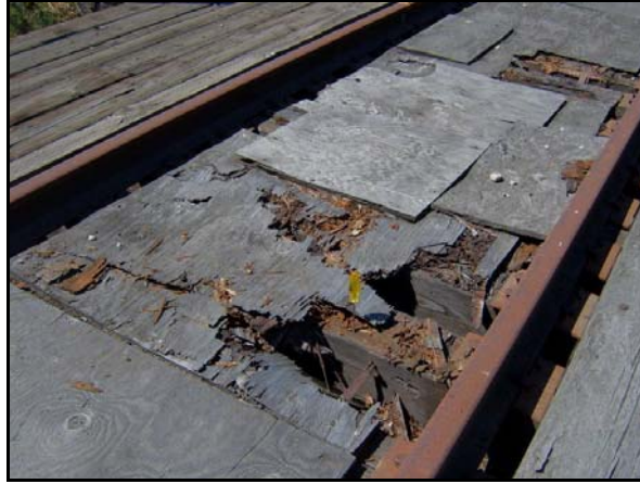
Figure 29. Deteriorated ties beneath the non-historic plywood. ( PAST Consultants, LLC Photo )
