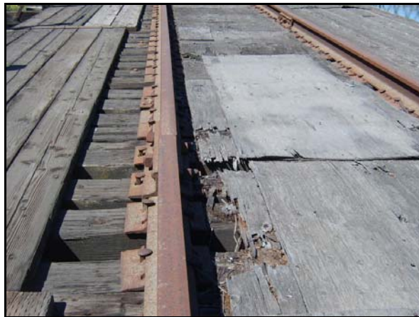
Figure 30. Typical view of rails and rail connecting plates. ( PAST Consultants, LLC Photo )
