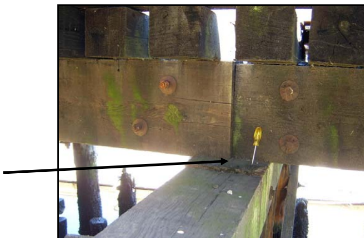
Figure 26. Typical wood deterioration where a pair of stringers meet atop the bent. The screwdriver is placed through a deteriorated shim (arrow) between the pile cap and the stringers. ( PAST Consultants, LLC Photo )
