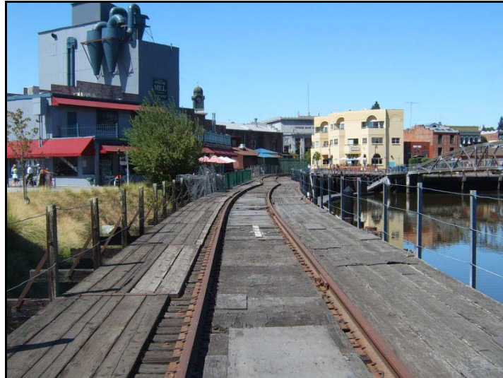
Figure 28. View of deck from east abutment, showing railings, ties, and non-historic deck boards and plywood. Note the bowed tracks at the top of the image adjacent to the McNear mill buildings, where slope instability and other factors have caused lateral movement of the Trestle. ( PAST Consultants, LLC Photo )
