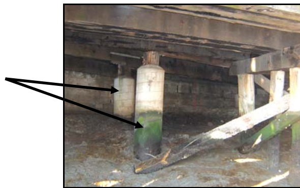
Figure 21. Example of piles wrapped in concrete, near the old McNear mill. (PAST Consultants, LLC Photo)
