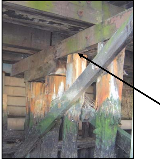
Figure 25. Various repairs at the pile tops, installed to level the bent. Repairs include an additional pile cap section installed over the two leftmost piles and shims installed on the right two piles, indicated with an arrow. (PAST Consultants, LLC Photo)
