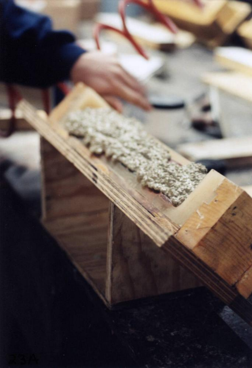
After curing for 45 minutes, buff-colored mix is poured to fill mold flush
